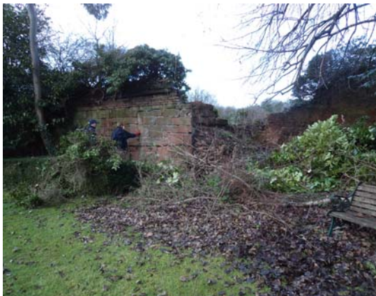
Urgent repair: The monastic wall to be rebuilt
